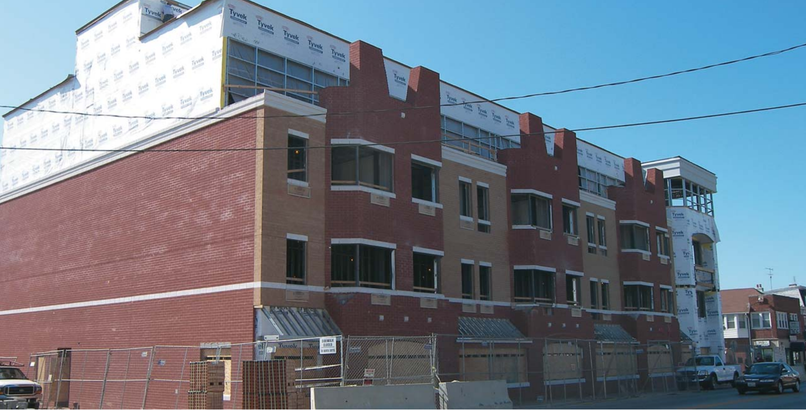
Construction on the Brandywine Health & Housing Center is expected to be completed in the spring of 2008.
